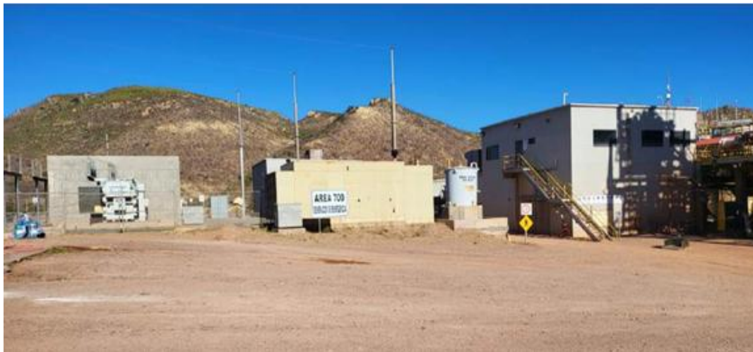
Figure 18-4: Diesel backup generator
