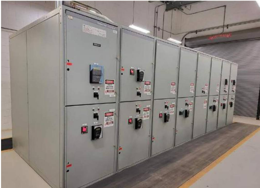
Figure 18-3: Site switchgear with two reserves
